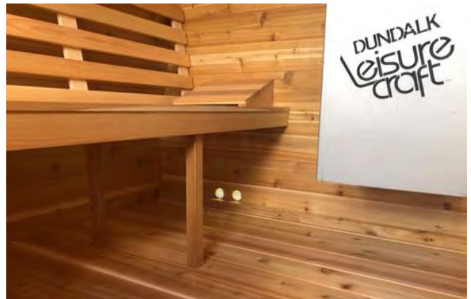
Inlet beside wood heater on Back wall
