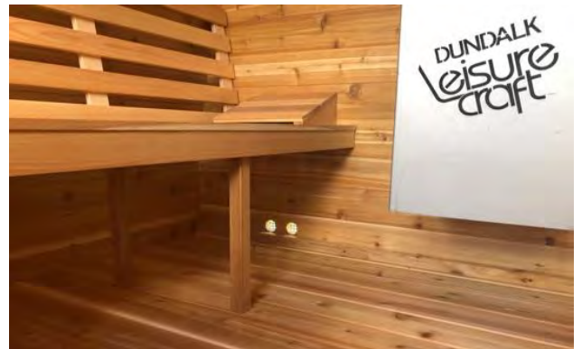
Inlet beside wood heater on Back wall
